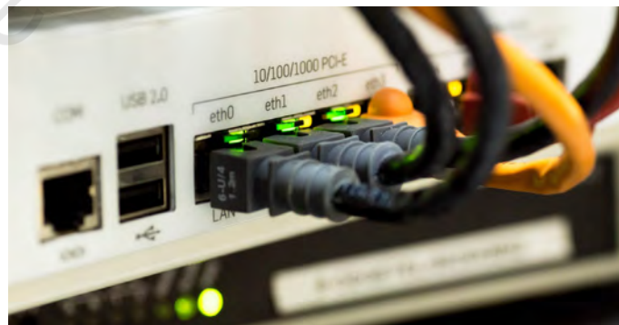
Figure 10.12: Cables connected to a network switch
